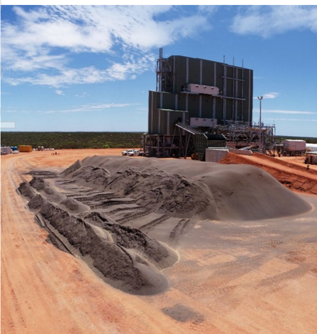
Figure 4 MSP Plant with HMC feed
